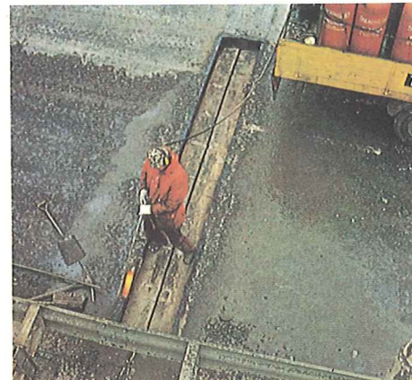
2. The resulting excavation is thoroughly cleaned and dried using a Thormack Hot Compressed Air lance.
