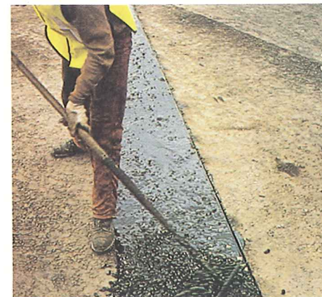
3. After coating all exposed surfaces of the excavation with Thormaseal BJ200, the surface is filled and made good with a controlled mix of hot single size aggregate and BJ200 compound.
