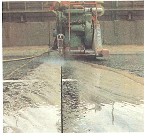
1. The existing surface is sawn and broken out to expose the concrete deck and expansion gap.
